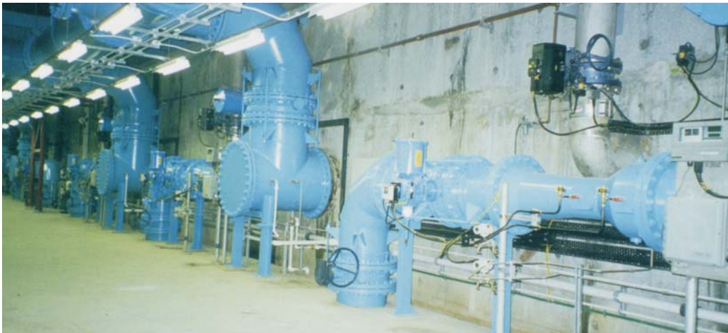
8-20" HVT-FC Halmi Flow Rate Controllers at the Siu Ho Wan WTP , Hong Kong, providing potable water for the new Hong Kong International Airport complex.
