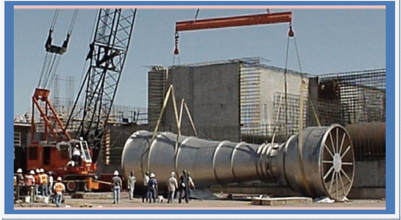
Worlds largest all 316L stainless steel, 180.0 inch HVT-FV venturi at the jobsite during installation.
